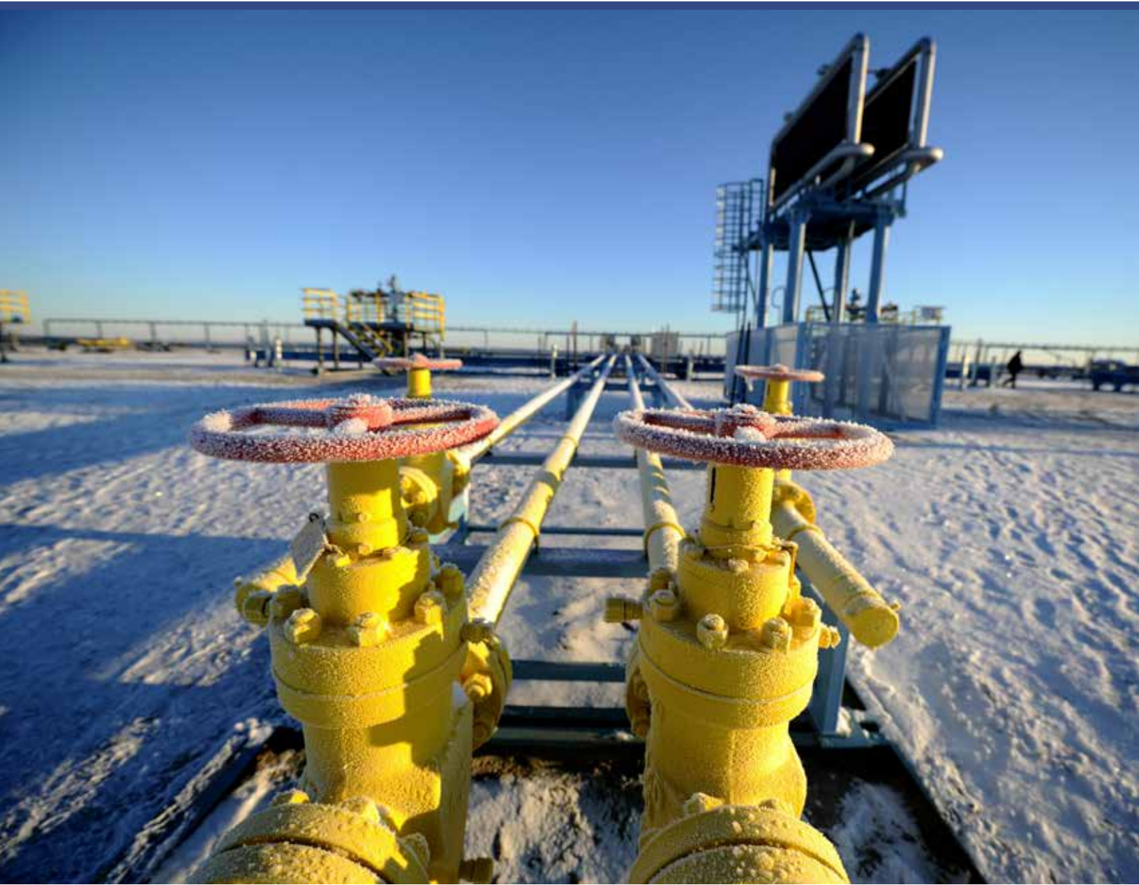
The site of wells cluster at the Bovanenkovo gas field. Photo: Stanislav Krasilnikov / TASS.
